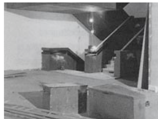
Silver gelatin prints showing the building during its transformation into the Tate Modern.
