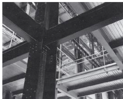
Silver gelatin prints showing the building during its transformation into the Tate Modern.
